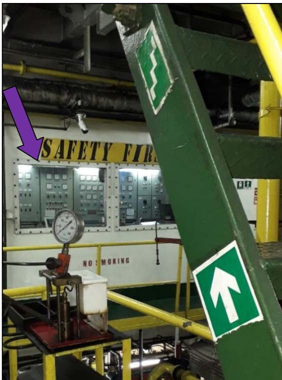
Figure 2: Engine control room window
