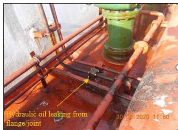
Figure 2: Photo showing location of the flange (photo taken after the repairs had been completed).
