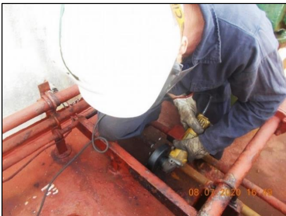
Figure 3: Simulated photo showing crew operating portable angle grinder on leaking flange.
