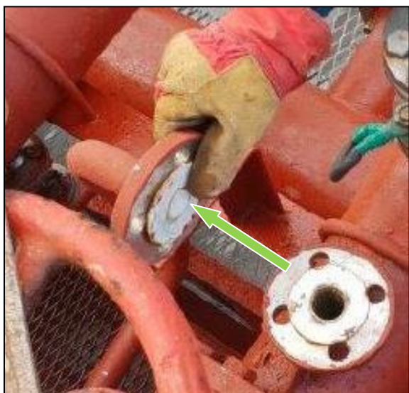
Figure 6: Cracked Teflon blank on the stripping line at the manifold's side
