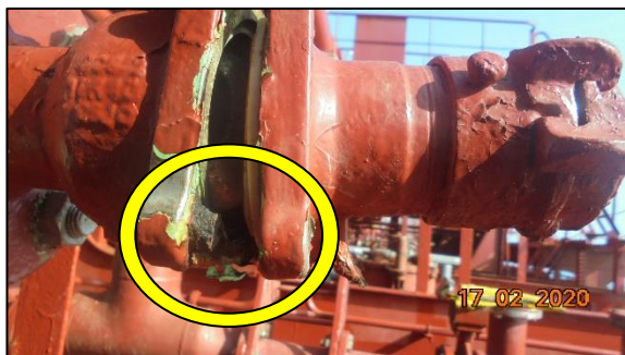
Figure 7: Close-up on the valve block, showing one of the ruptured bolts (circled in yellow)
