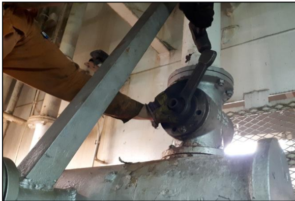
Figure 2: Simulation to show how the sight glass was being tightened
