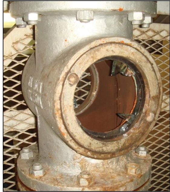
Figure 3: Damaged sight glass after the accident
