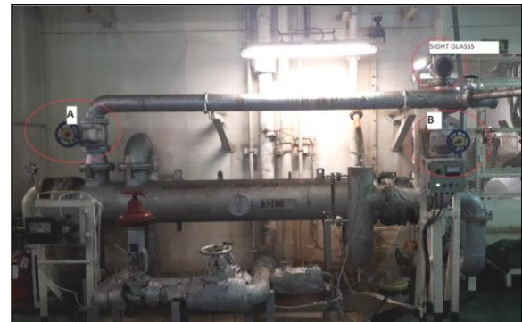
Figure 6: Location of the valves and sight glass
