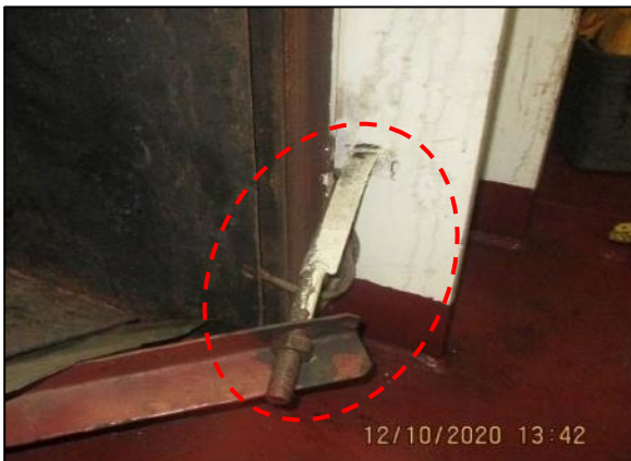
Figure 7: Securing arrangement which gave way
