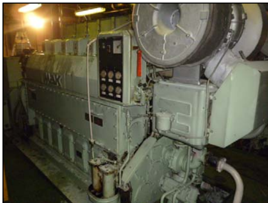
Figure 6: Location of generator instrumentation panel
