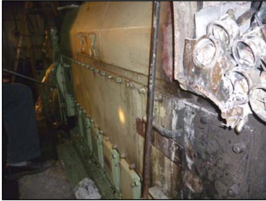
Figure 2: Extent of fire damage did not reach the prime mover units
