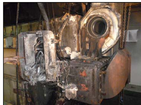
Figure 1: Localised damage restricted to turbocharger and intercooler area
