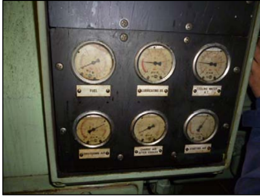
Figure 5: Instrumentation panel on one of the other intact generators
