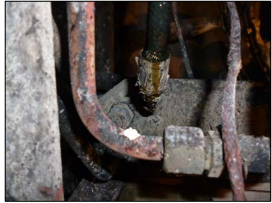
Figure 4: Leaking armoured flexible rubber hose fitted to the fuel gauge of no. 3 generator
