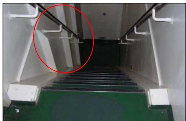
Figure 6: Aft section stiffeners protrude towards the stairway
