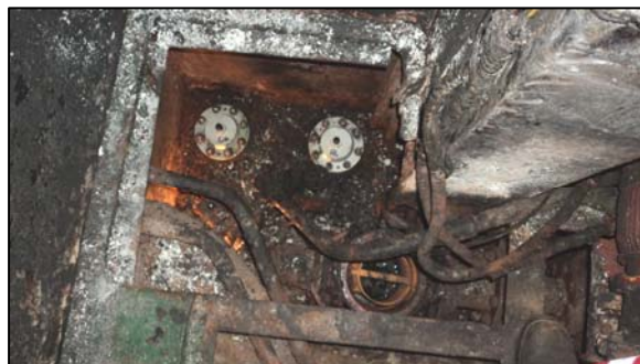
Figure 4: Fire damage inside the emergency fire pump space
